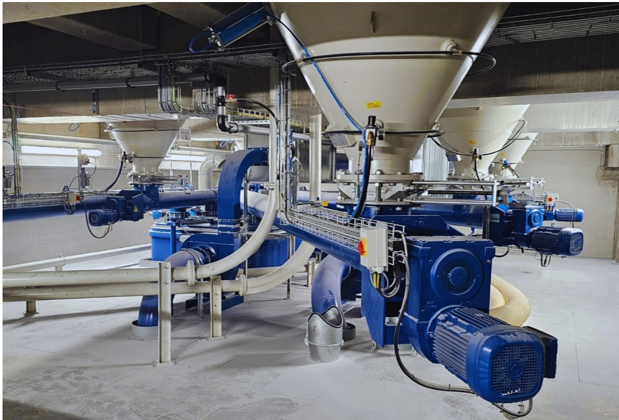
Silo discharge of raw materials for the mixing process at KLB.
